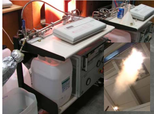
Fig. 3: Hydronic 2x15kW H 2 /O 2 Steam Generator in the parallel mode. Exhaust of superheated steam.
